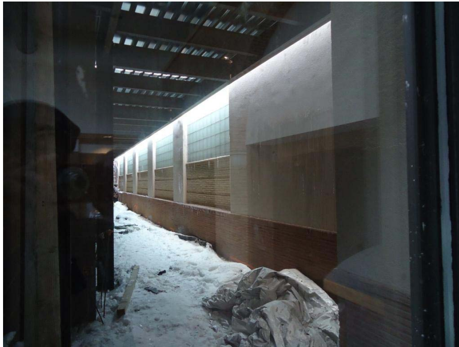
Photo 1 - View of South Windows to be removed during Phase II Window Putty Containing 20% Chrysotile Asbestos.
