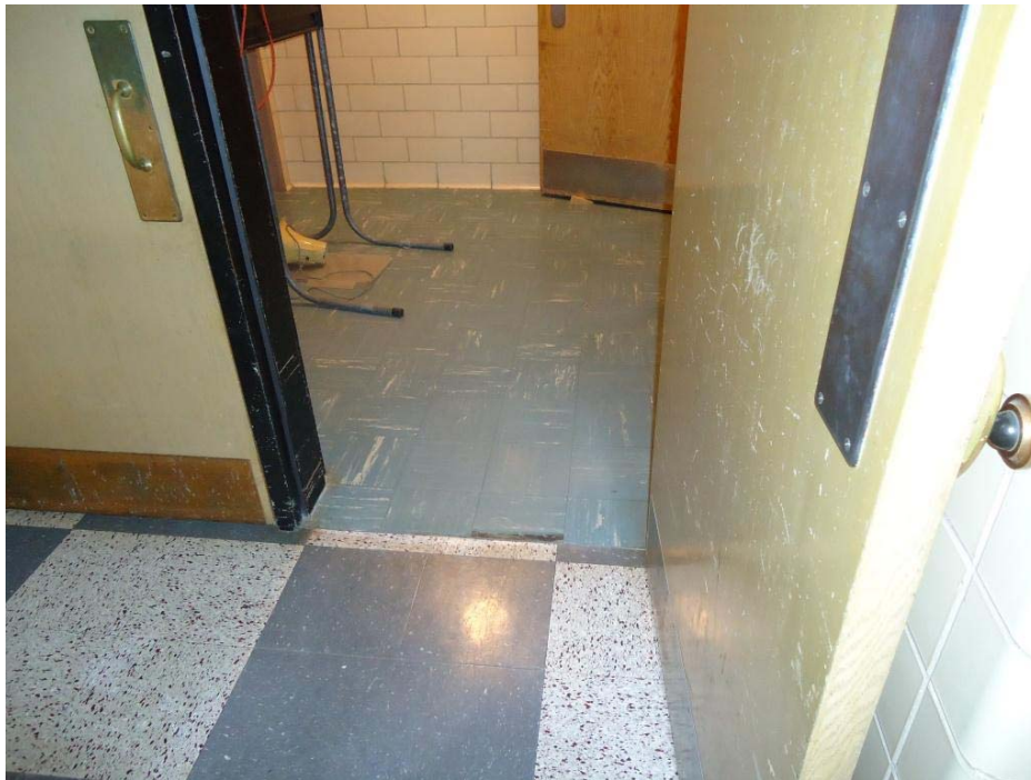
Photo 4 – View of 9-inch Floor Tile at Entrance to Women's Locker Room. Floor Tile 6% Chrysotile, Mastic 4% Chrysotile.
